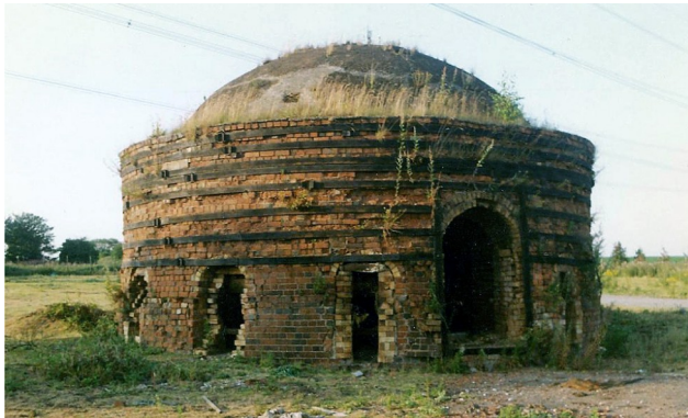
Photograph of the derelict Shenstone 'beehive' kiln showing access and fire holes. The chimney had already been demolished.
